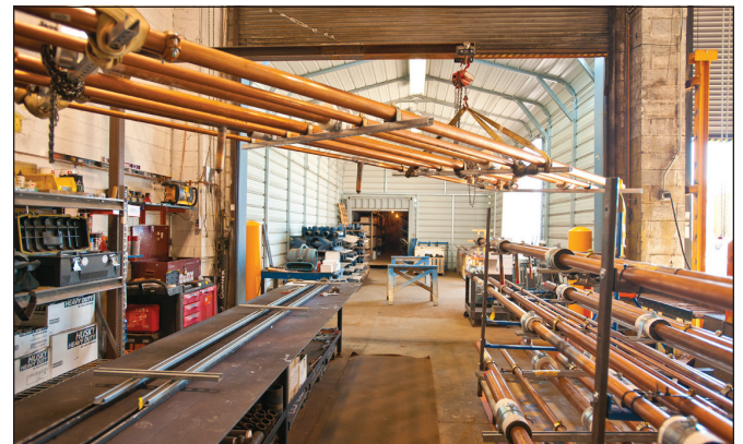
Figure 2. Prefabricated Racking of Services: prefabricated racks in the service corridor that includes all major utilities and services.
